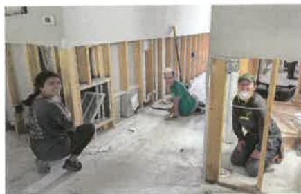
Students help remove damaged baseboards and drywall from a home in Fletcher, North Carolina.
